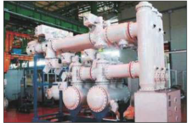
170kV GIS : 3-Ph Enclosed Busbar
